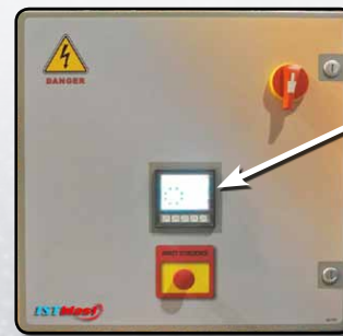
HMI* touchscreen control
