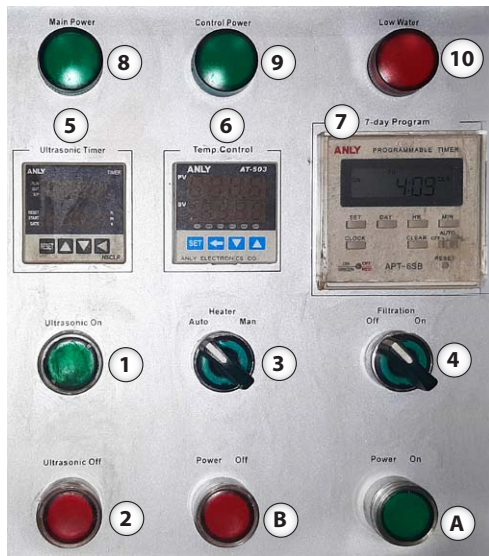
TANK CONTROL PANEL (IN FRONT)
